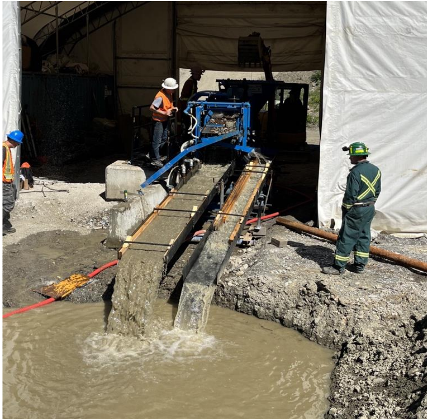
Backend of Wash Plant – Boil Boxes
